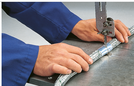
Position conduit at right angle to the band saw and carefully cut through the conduit
