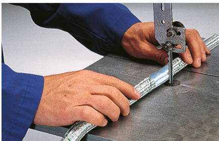
Bind conduit with metal adhesive tape at the cutting position 2 or 3 times
