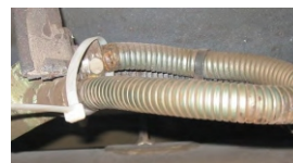
PVC Jacket Degrades Limited Service Life
